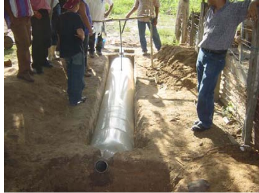
Installation of the plastic biodigester unit as part of the waste water treatment plant
