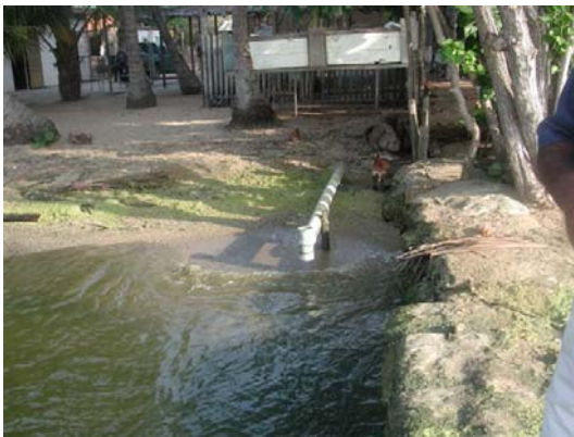
“Black water” pipe lines going directly to the Maracaibo Lake
