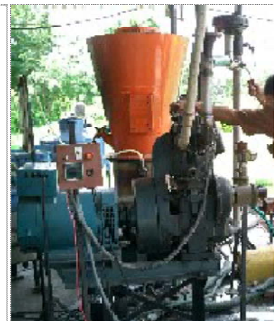
Figure 9: Small scale gasifier-engine in India (Source: ANKUR 2003)
